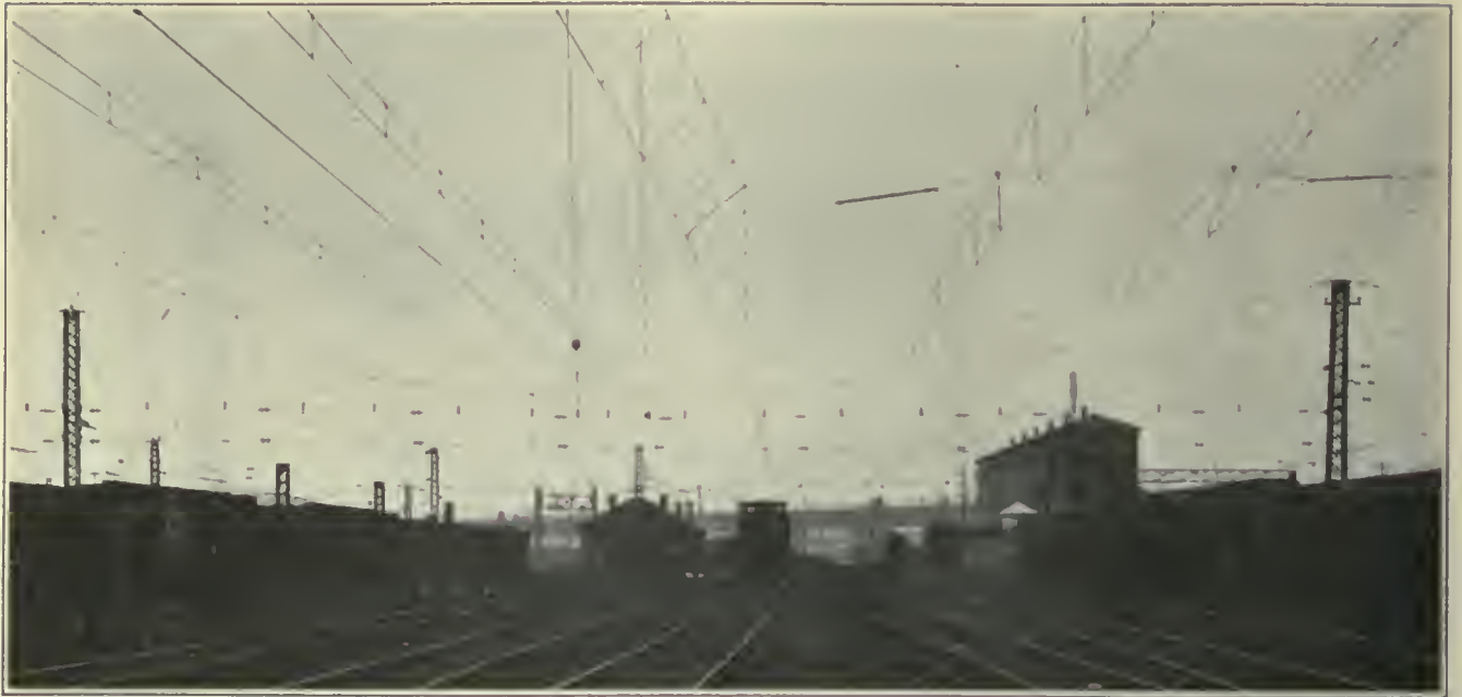
FIG. 521. OVERHEAD CONTACT SYSTEMS. Yard Track Construction. 11,000-Volt Single-Phase Electrification, Harlem River Yard, New York, New Haven & Hartford Railroad
